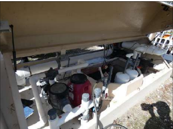
Pool Pumps and Equipment
