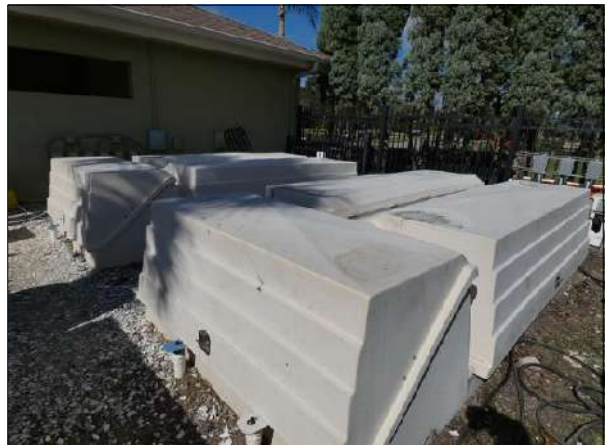
Pool Equipment Housing Boxes
